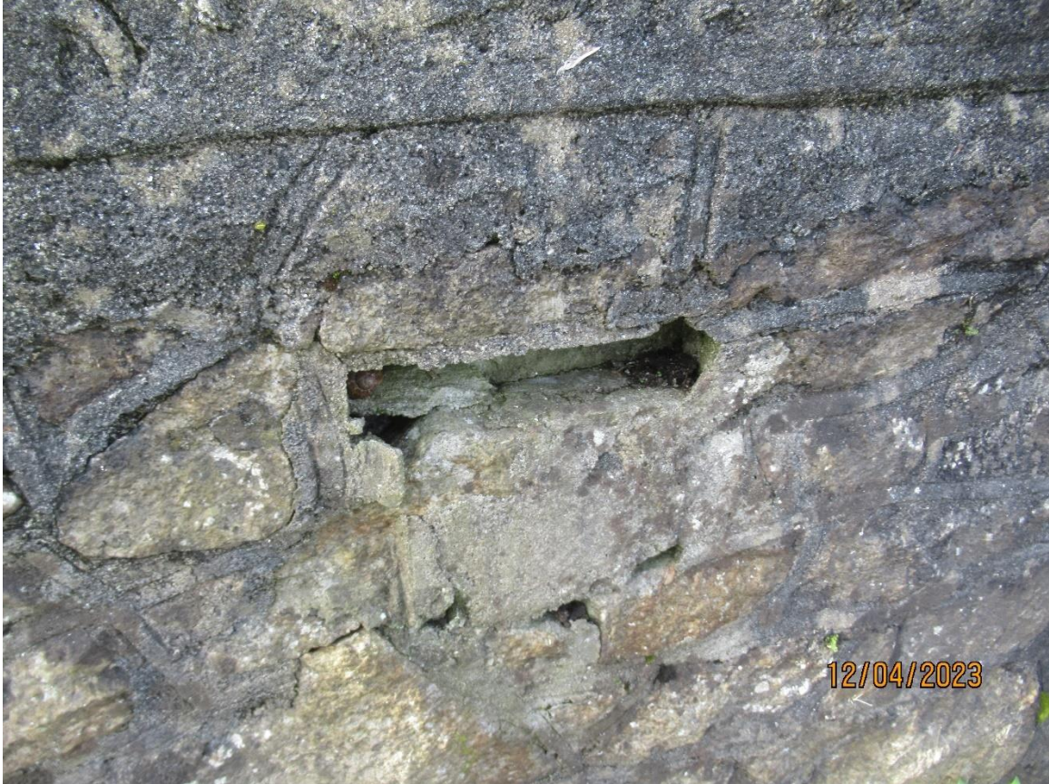
P3 – vegetation and poor jointing
