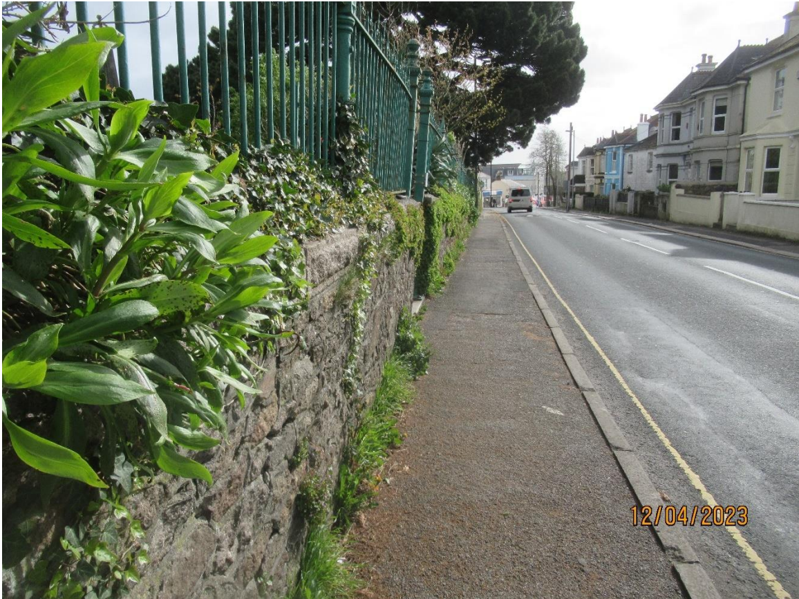
P6 – displaced west end of south boundary wall
