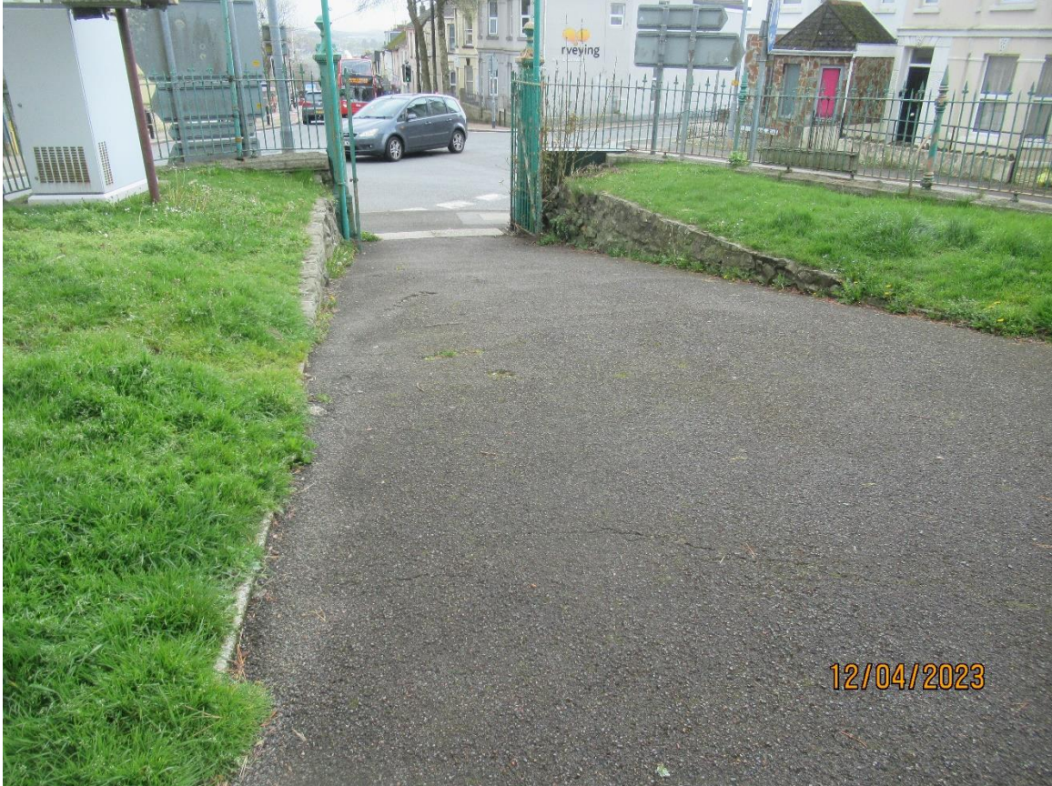
P20 – cracked path
