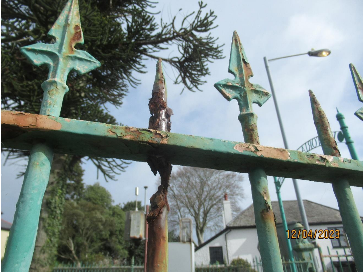
P15 – corroded St Stephens Road railings
