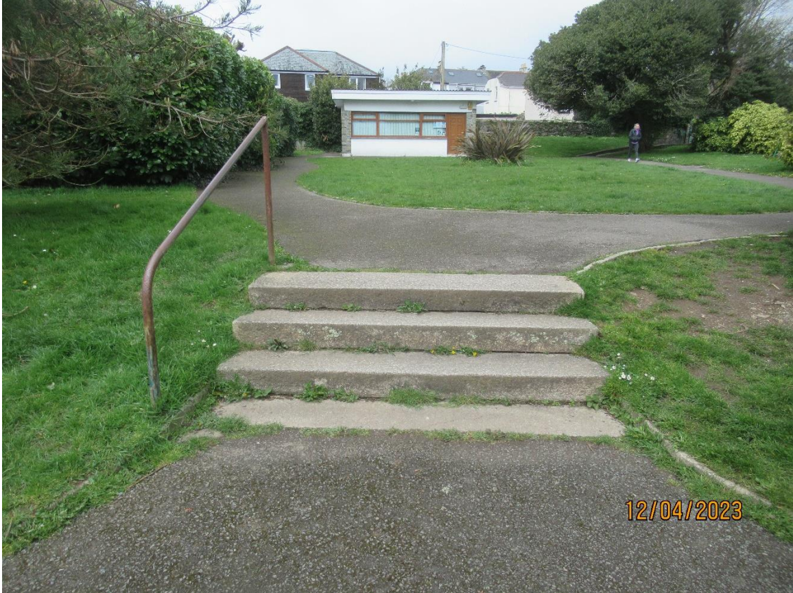
P19 – handrail east of Maurice Huggins room
