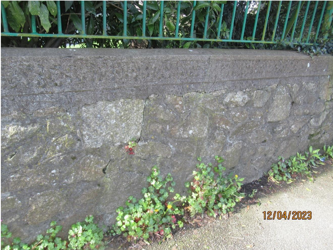
P2 – diagonal crack in wall
