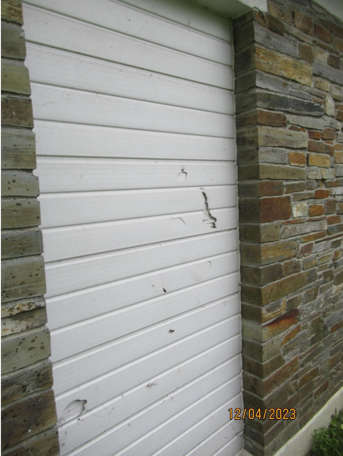
P25 – damaged fascia panels
