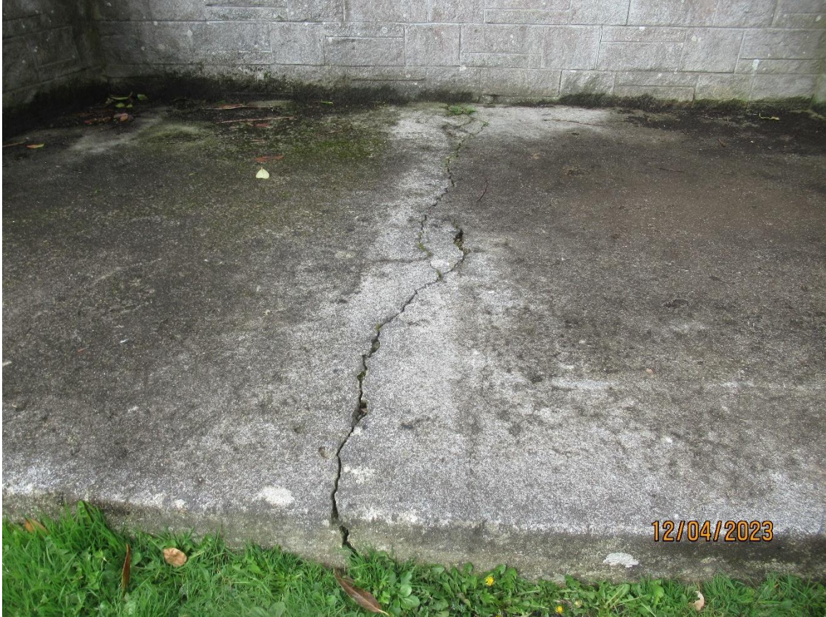
P21 – cracked floor slab to bandstand
