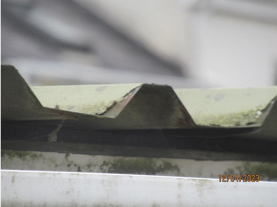
P24 – corroding sheet edges
